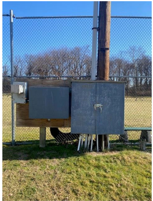
Orchard Ave Lighting Panels (Same panels as location 3A)
