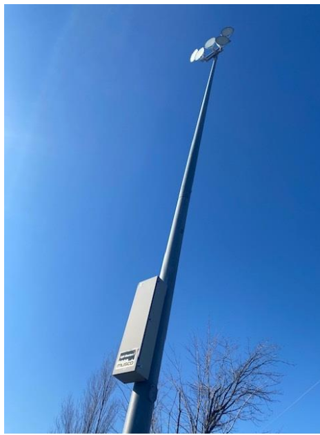
Softball Lighting Pole
